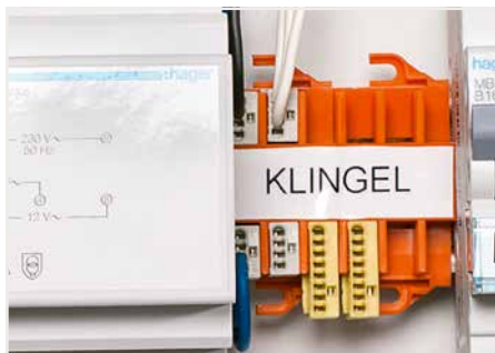
DIN-35 rail-mount application (residential door bell)
