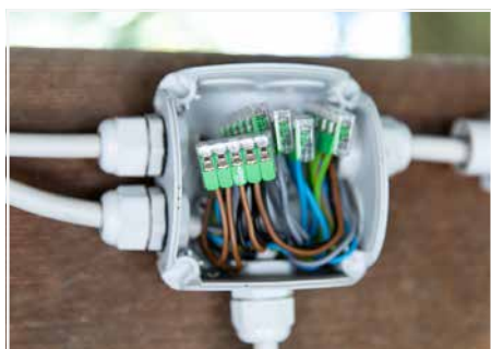
Wiring in a distribution box
