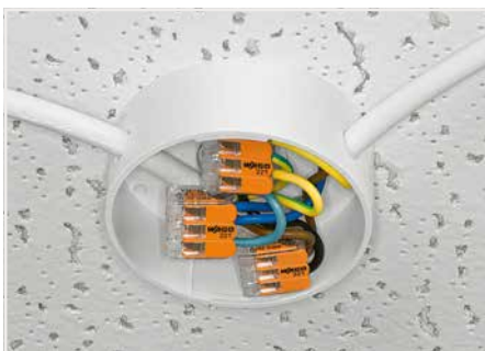
Lighting distribution in a ceiling canopy
