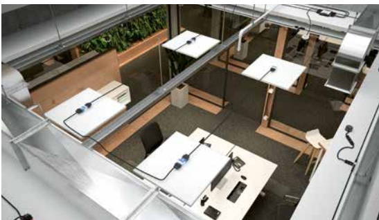
In suspended ceilings
